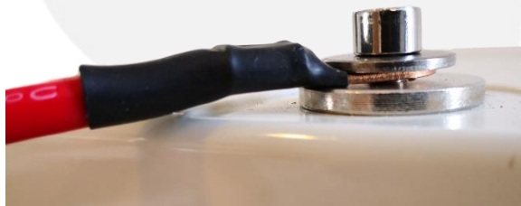
Figure 4. WRONG! Loose connection by using too long bolt
